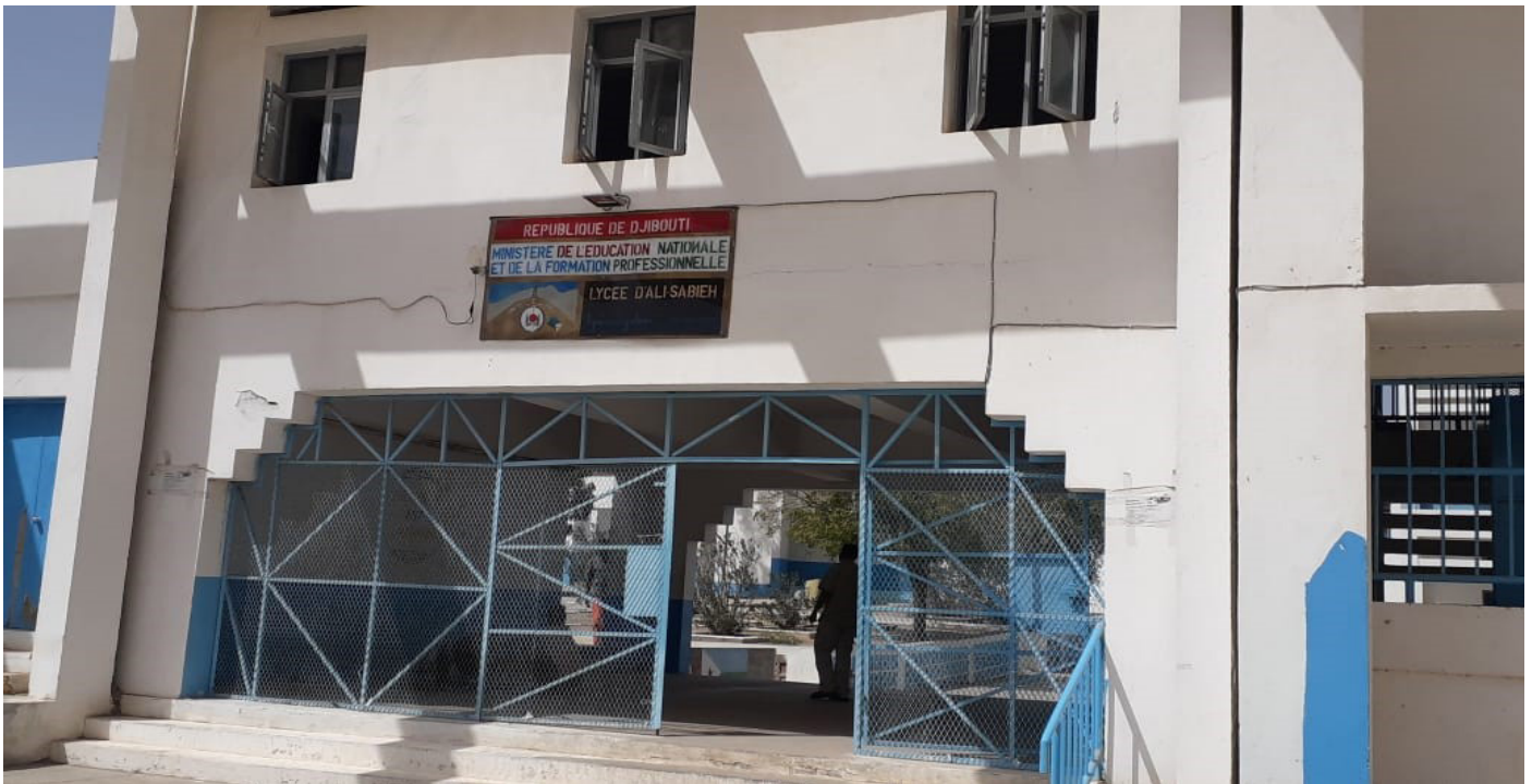
The Lycée Technique vocational and technical training college in the Ali Sabieh region will be upgraded as part of Investment Window 2, which focuses on skills development.
